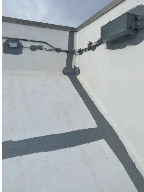
AGED & WEATHERED ROOF
