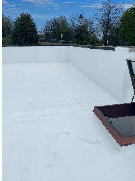
AGED & WEATHERED ROOF
