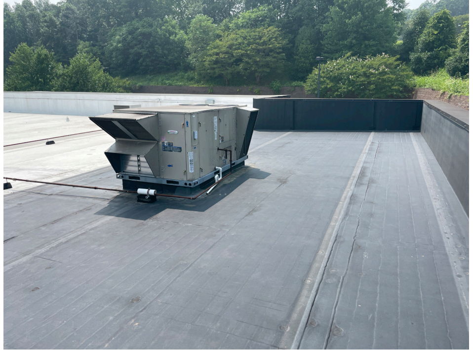
AGED & WEATHERED ROOF
