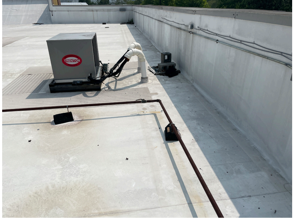
AGED & WEATHERED ROOF
