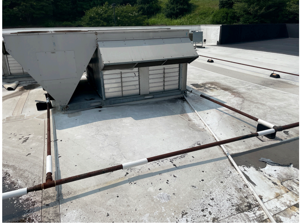
AGED & WEATHERED ROOF
